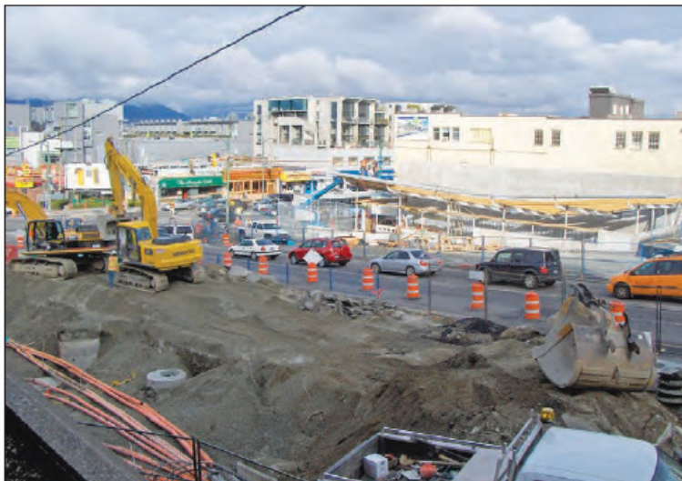
In transit: major projects such as the Canada Line (shown here at Cambie and Broadway) may be wrapping up this year, but recent reports indicate that non-residential construction holds some of the best prospects as the economy heads south
